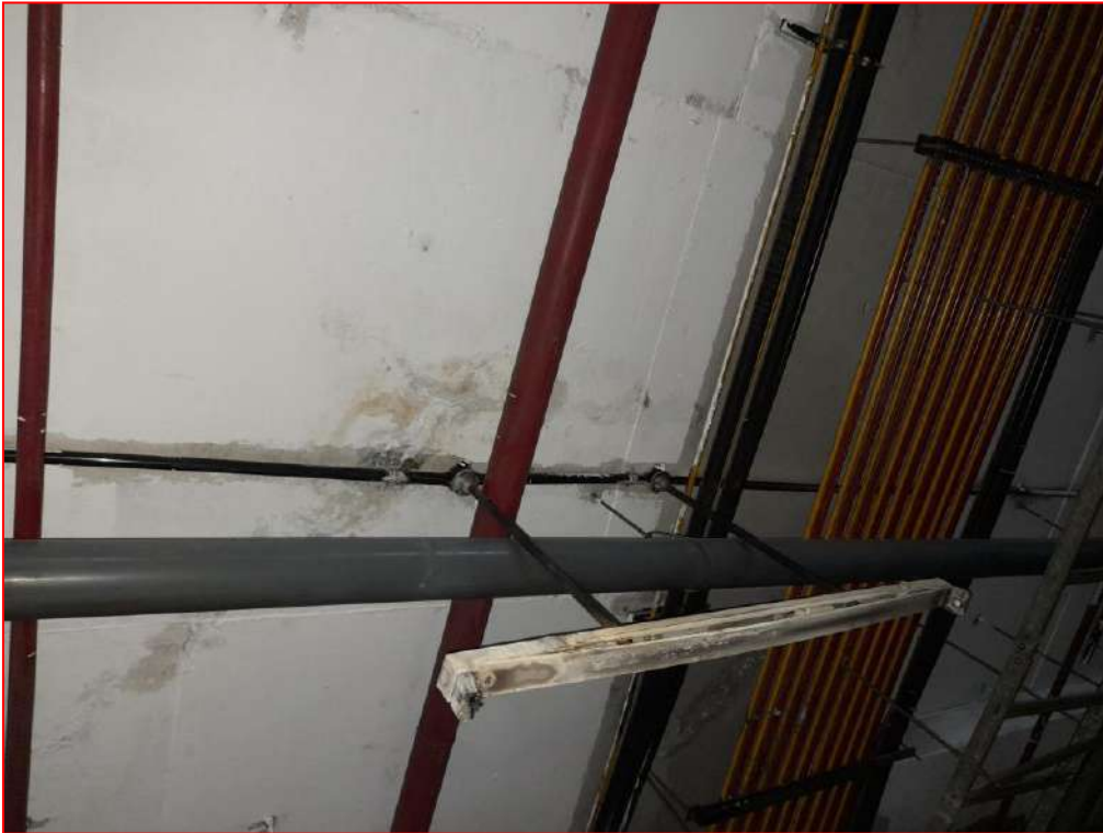
Seepage marks on ceiling.
