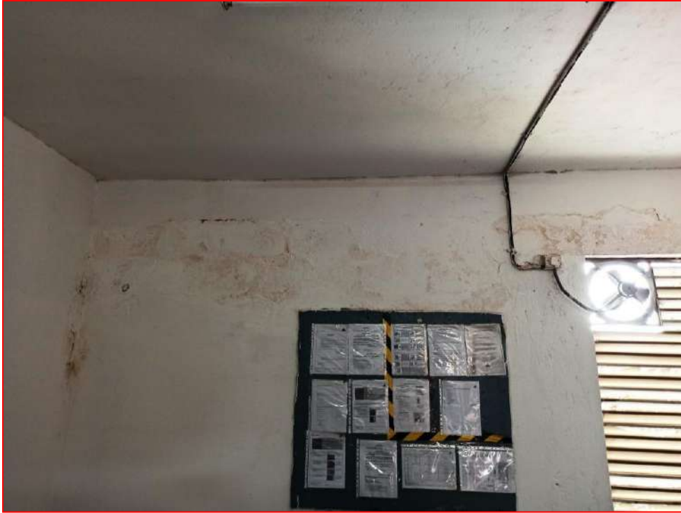
Seepage marks were found on wall of LMR.
