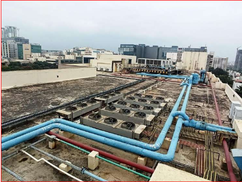
View of various service pipe lines run on terrace surface with the support of concrete pedestal.
