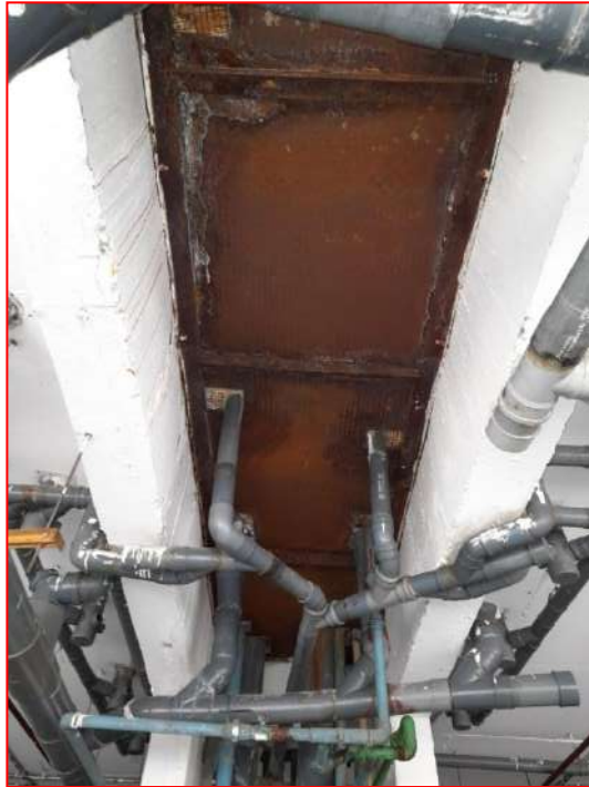
Plumbing duct chequered plate observed corroded.
