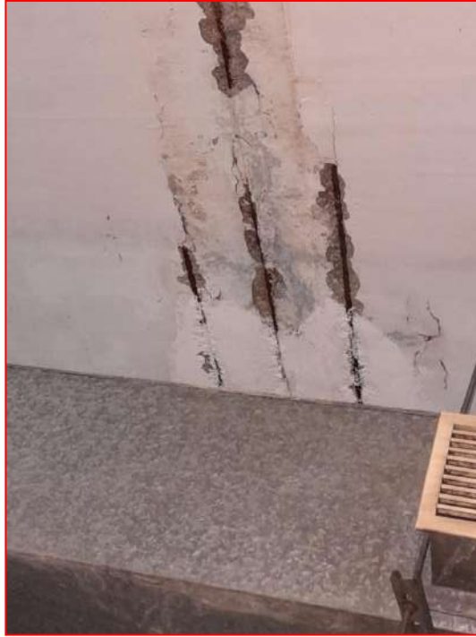
Reinforcement exposed observed on ceiling.
