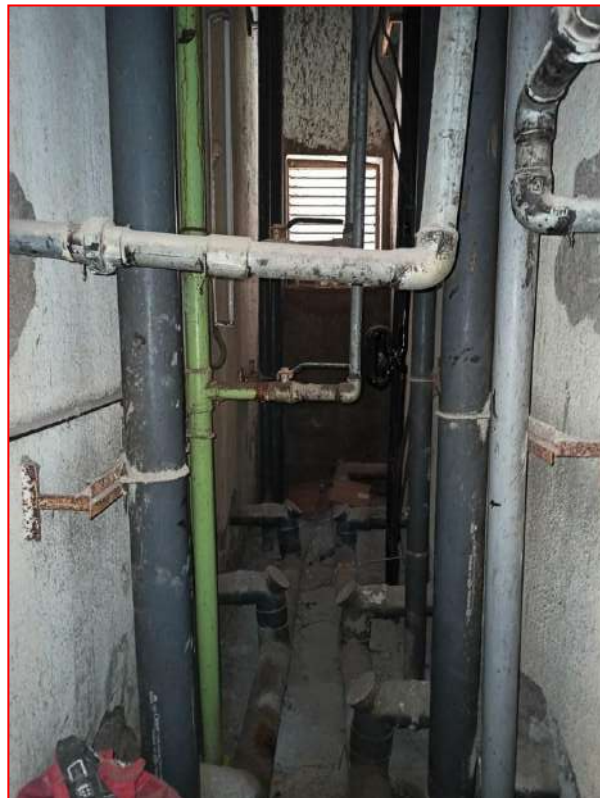
View of Plumbing Duct consist Drain & water supply pipe lines.
