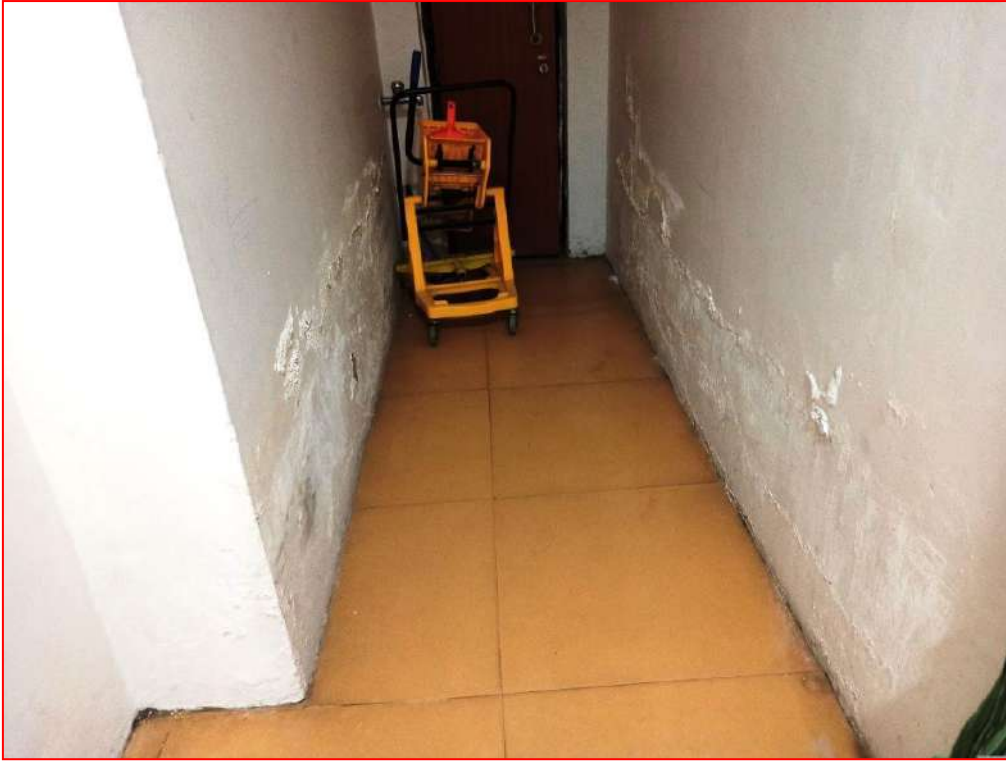
3 rd floor level: Dry seepage marks observed on walls.
