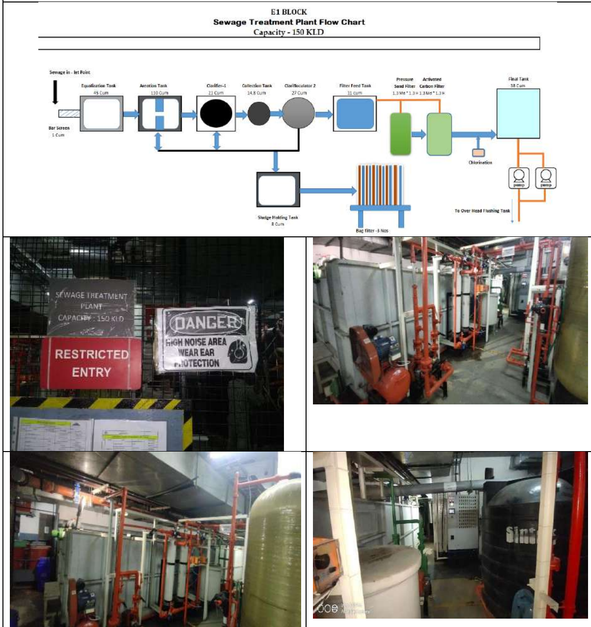
Figure 13: Flow chart and photograph of the E1 Block STP: 150 KLD
