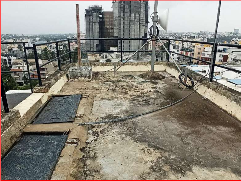
View of damaged and discolored IPS above overhead tank.
