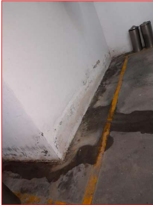
Common toilet observed water seepage.
