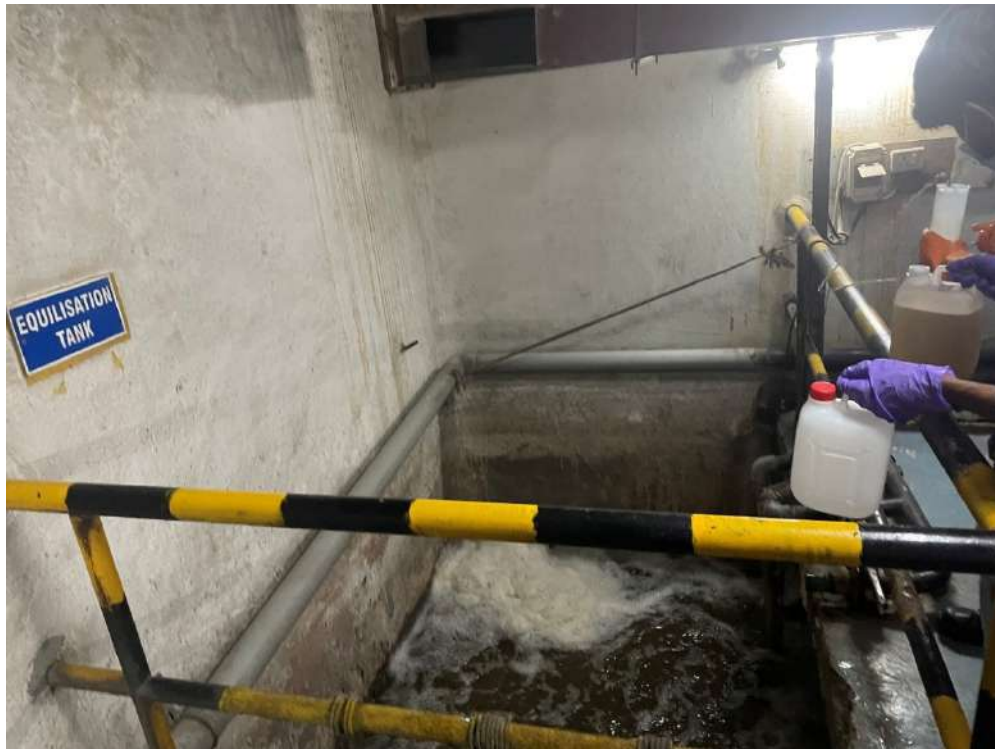
Figure 3: Photograph of sampling of the treated water on the site
