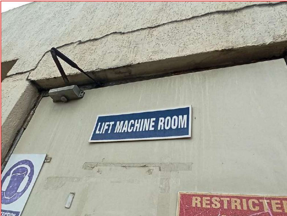
Lintel beam above lift machine room was observed with cracks.
