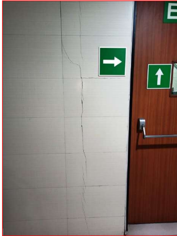
2 nd floor level: Separation crack were found on wall near the fire exit staircase.
