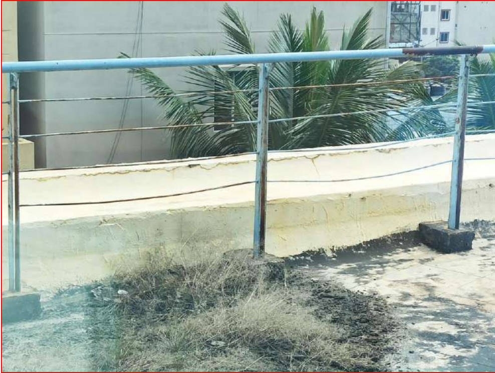
4 th floor level: Vegetation growth were observed at terrace level.
