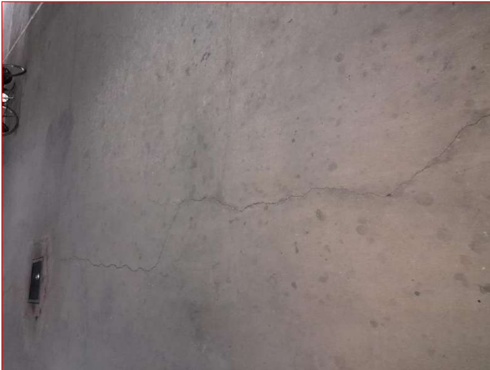
IPS finished flooring observed cracks.
