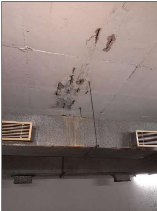
Reinforcement exposed observed on ceiling.
